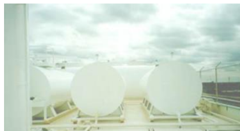
Figure 7-3: Shop-built containers elevated on saddles.
