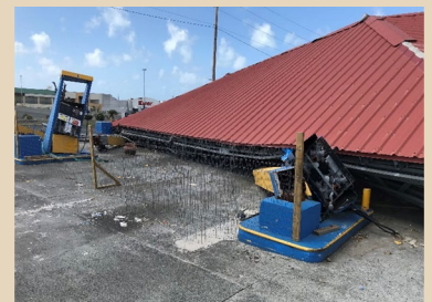
Destroyed dispensers after Hurricane Maria, 2016. Credit: EPA
