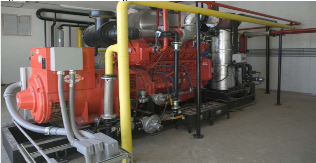
Figure 9 – Guascor 300kW Engine Generator Set
