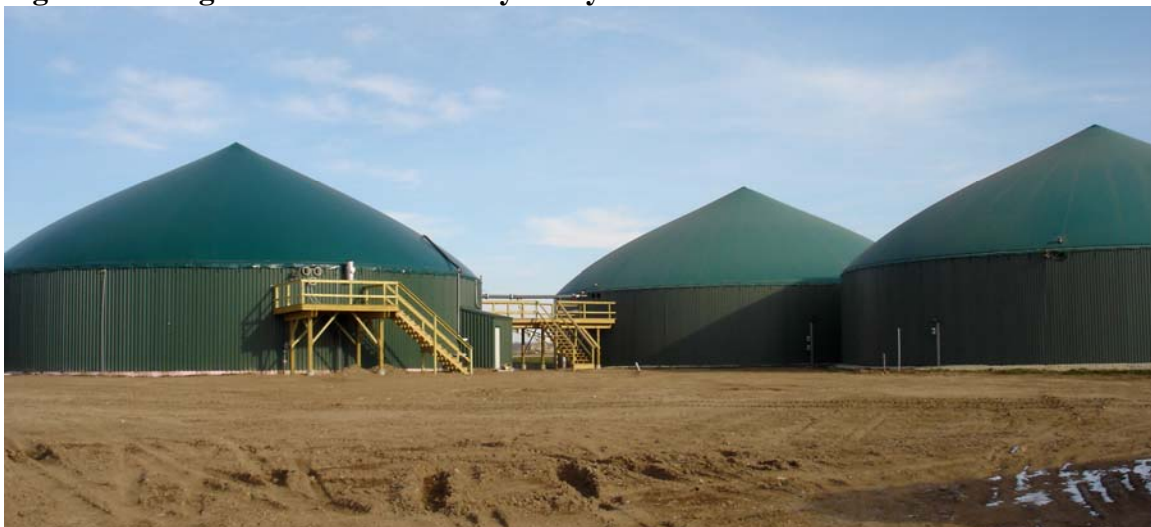
Figure 24 – Digesters at Green Valley Dairy
