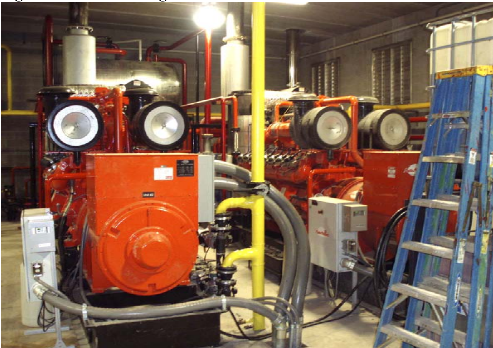
Figure 27 – Holsum Engine Generator Sets at Elm Road
