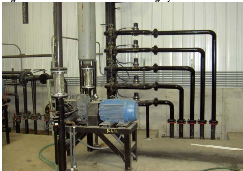
Figure 48 – Statz Brothers Gas Mixing System
