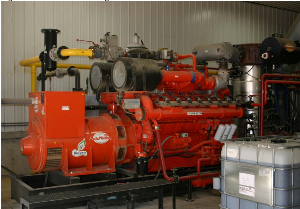
Figure 49 – Statz Brothers Engine Generator Set
