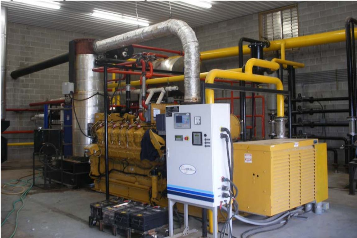
Figure 43 – Pagel’s Ponderosa Engine Generator Set
