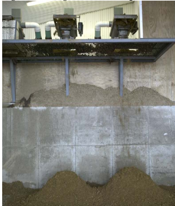
Figure 35 – Digested Solids Separation Area
