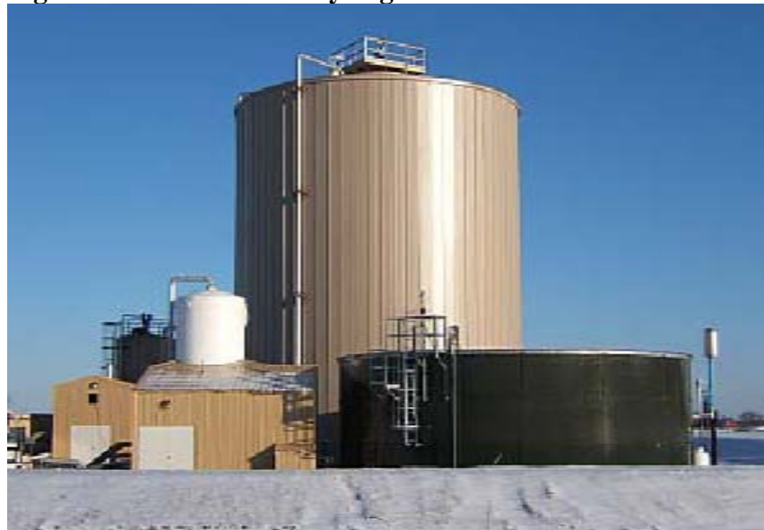
Figure 22 – Five Star Dairy Digester
