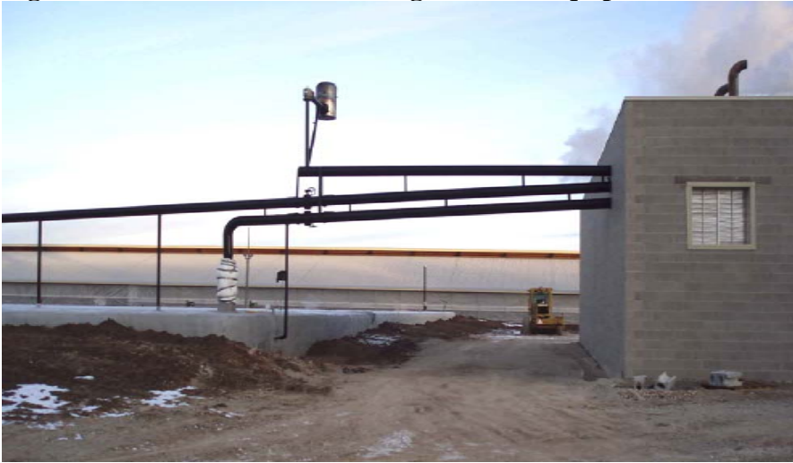
Figure 26 – Holsum Elm Road Digester and Equipment Shed
