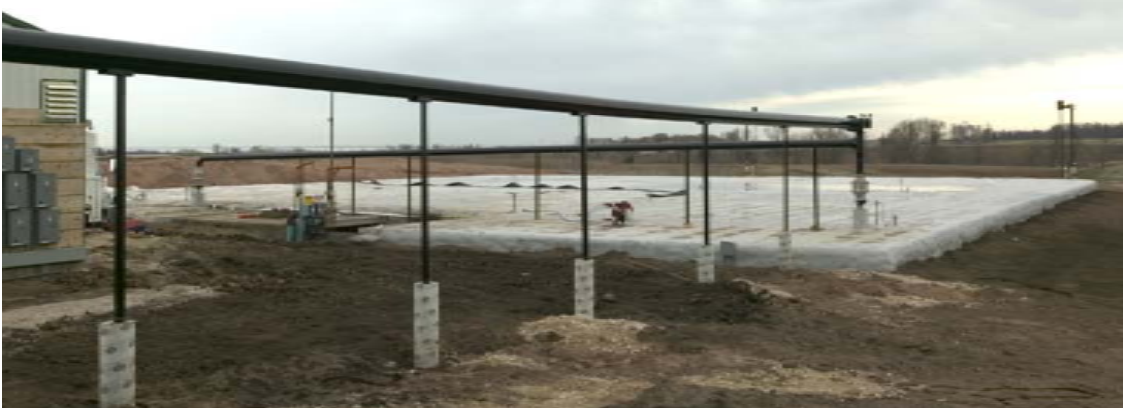
Figure 32 – Digesters at Lake Breeze Dairy
