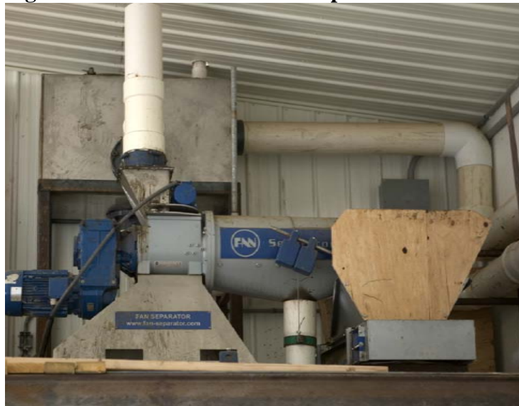
Figure 46 – Screw Press Solids Separator
