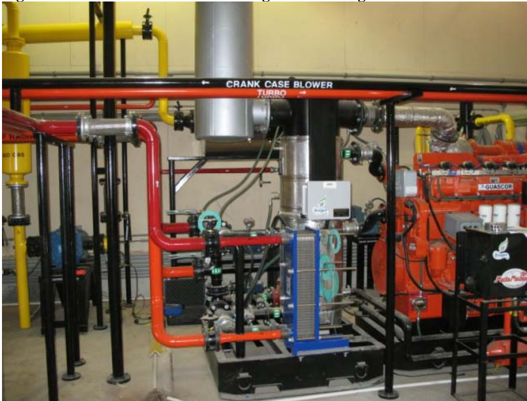
Figure 61 – Volm Farms Heat Exchanger for the Engine Generator Set
