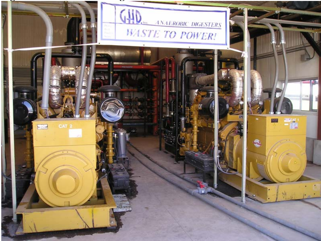
Figure 33 – Lake Breeze Engine Generator Sets
