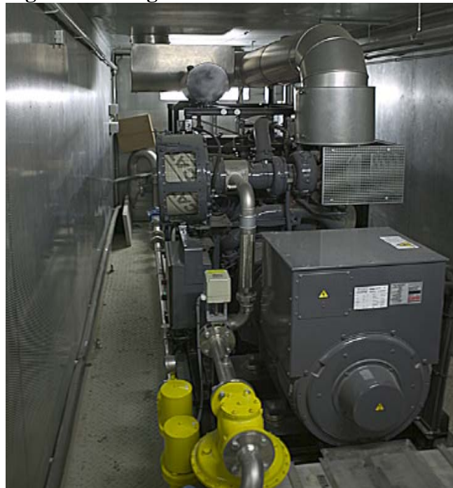
Figure 57 – Engine Generator Set in Container
