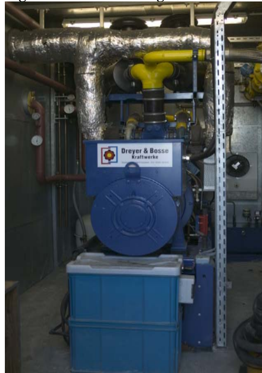
Figure 53 – Sunrise Engine Generator Set
