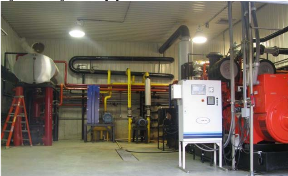
Photo courtesy of Norm-E-Lane
