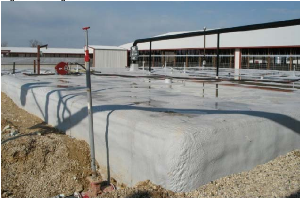
Figure 60 – Digester at Volm Farms
