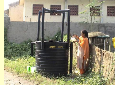
India: household biogas System
