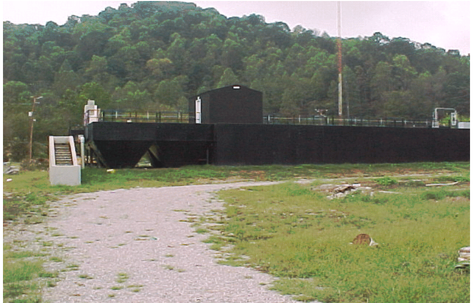
Figure 3: Package Plant, Hindman, Kentucky
