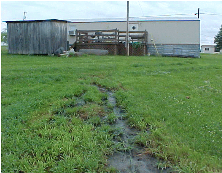
Failed Septic System: Preston, KY
