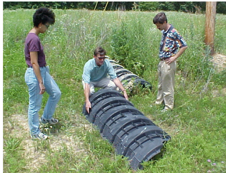
Infiltrator Drainage System: Preston, KY
