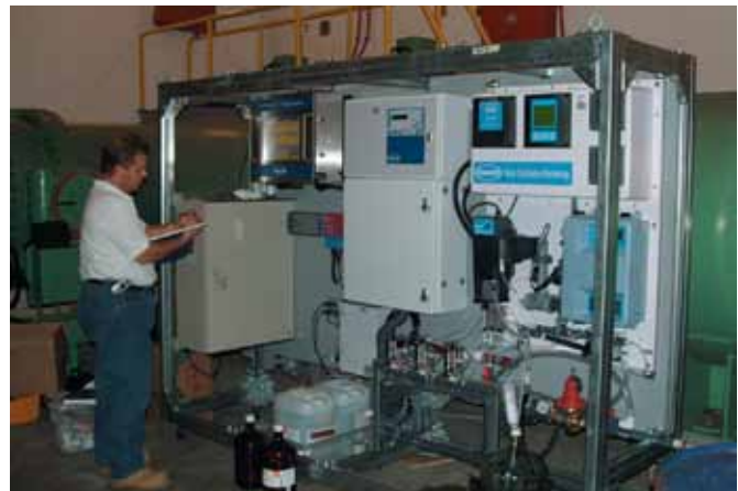
Figure 2.12 First Pilot Utility - Water Security Initiative Instrument Panel Type A
