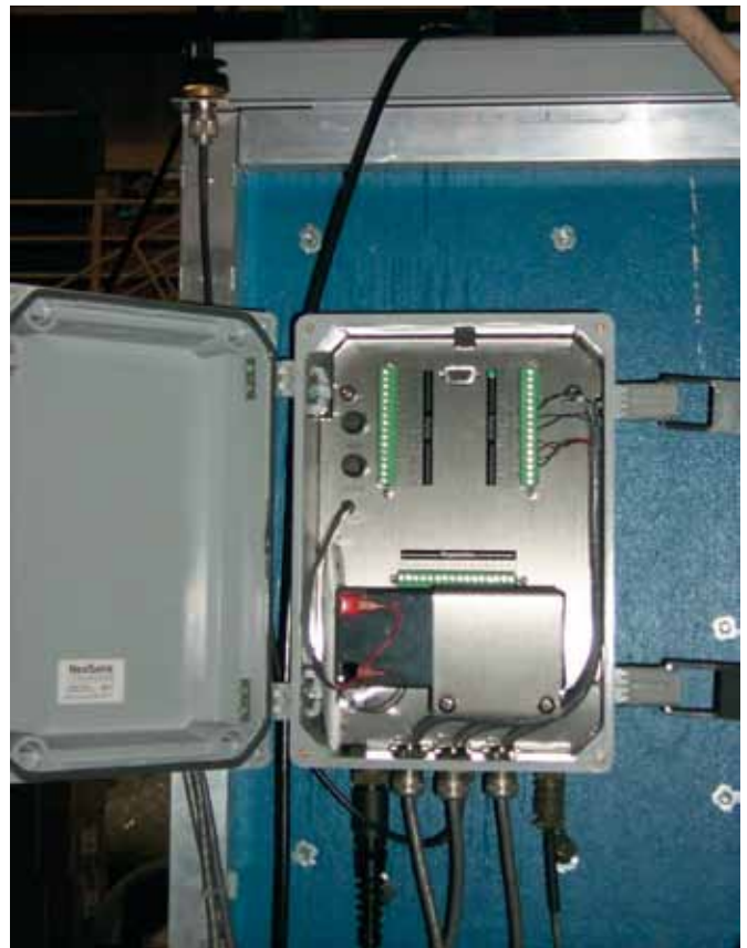
Figure 3.4 Field Communications Enclosure.
