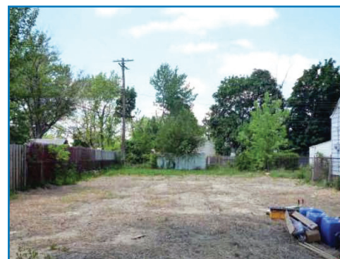
Debris left behind after demolition makes site restoration much more difficult.
