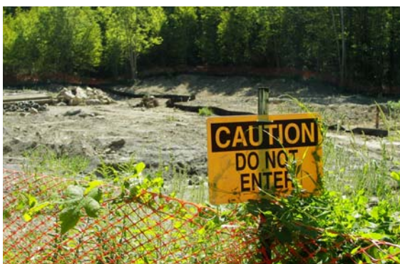
A caution sign at the Ringwood site (EPA OIG photo taken August 2006).
