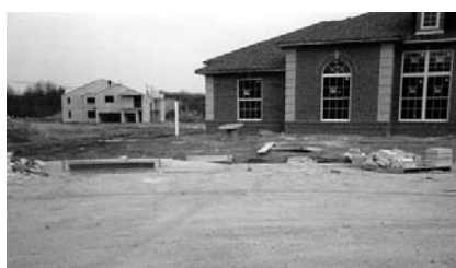
Improperly managed construction sites can clog estuaries with tons of sediments (photo by R. Ohrel).
