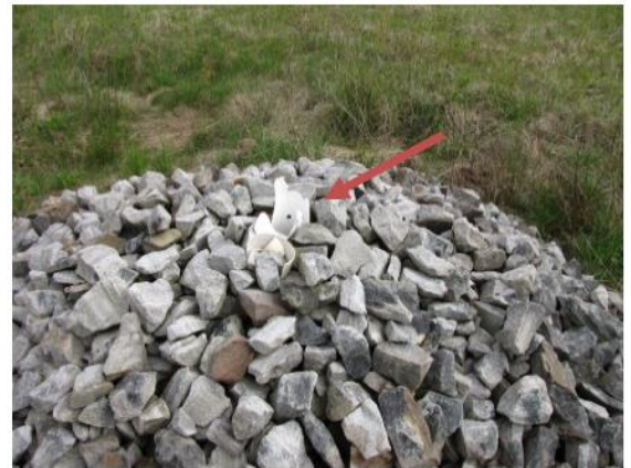
Protective rock mound installed around a damaged gas vent (see arrow) at the Lackawanna Refuse site. (USGS Photo.)
