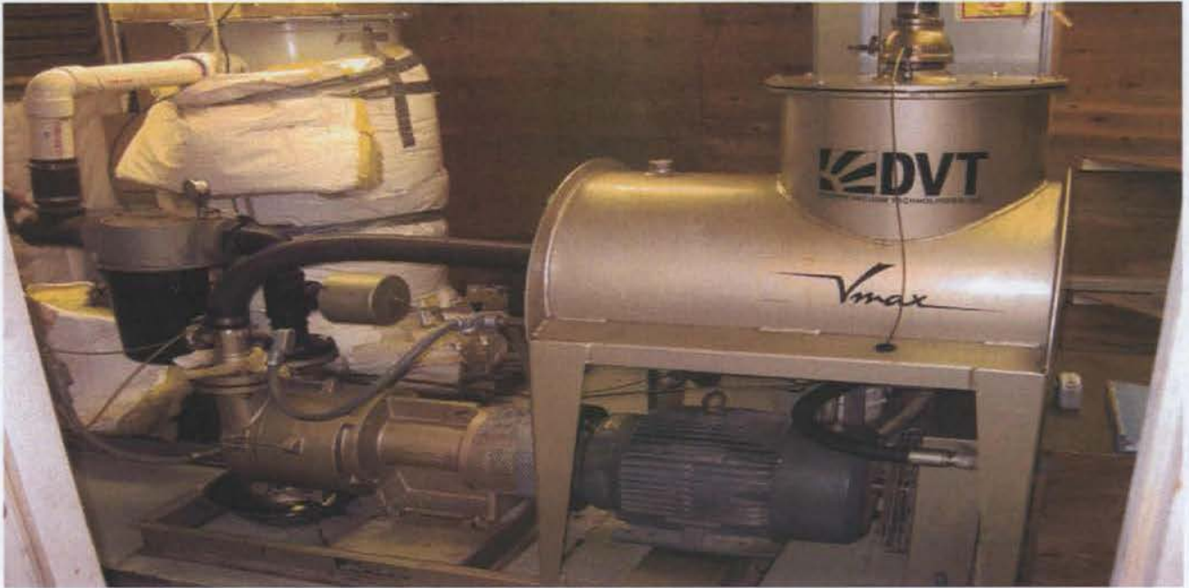
Photo 3 – Soil Vapor Extraction System blower.
