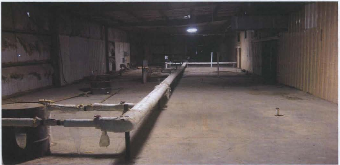
Photo 4 – Soil Vapor Extraction System Wells (Area B)
