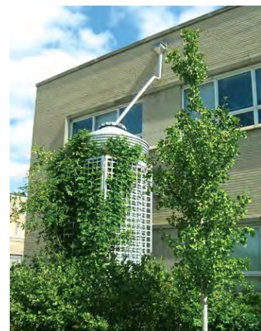
Chicago's Green Permit Program reviews permits much faster for projects that include LID practices like this cistern at the Chicago Center for Green Technology.
