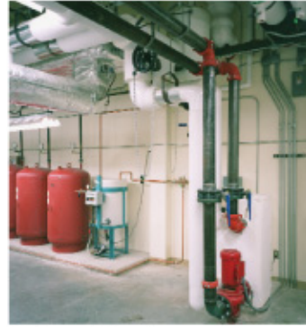
A plate and frame heat exchanger system was added to the initial design after energy modeling revealed additional energy efficiency opportunities.
