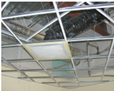
During construction, the HVAC system and duct work were sealed on a daily basis to prevent infiltration of any dust, chemicals, or odors due to construction. Before occupancy, the system was flushed and fresh air filters were added.
