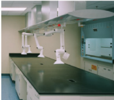
Sophisticated variable air volume (VAV) fume hoods and systems allow ventilation, cooling, and heating requirements to be reduced when hoods are closed, at night, and on weekends.
