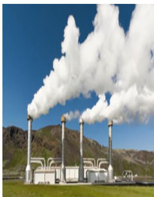
A geothermal plant, part of a greenhouse gas reduction project. (U.S. Department of Energy photo)
