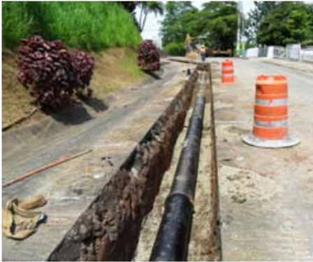
Pipes at the Las Marias Potable Water System Phase IIA construction site. (Photo courtesy Constructora De Aguada, Inc.)
