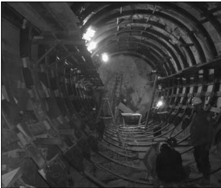
The City of Richmond, VA won a National CSO Control Program Excellence Award in 1999 for its efforts to control CSO discharges, which include the construction of deep tunnels for storage, as shown.
