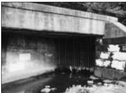
EPA collected permit number, information on the number and location of outfalls, and requirements for CSO controls for all CSO communities. This information was supplemented with municipal case studies to capture the varying degrees of progress in CSO control implementation.
