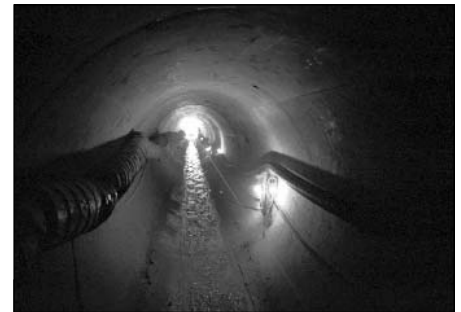
Region 2 tracks and oversees state CSO programs. The State of New Jersey conducts the inspections of CSO facilities, including this new separated sewer tunnel in New Brunswick.
