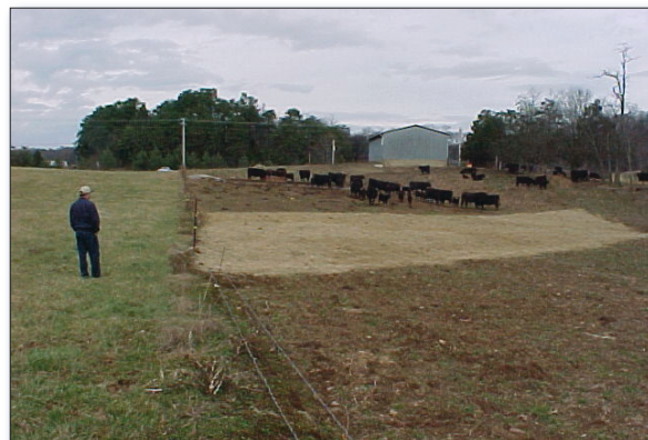
Figure 2. Landowners installed heavy-use area protection to stabilize the land and control erosion.
