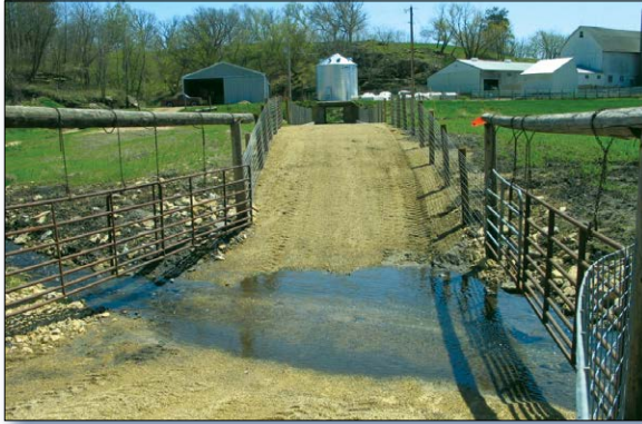
Figure 2. Project partners worked with a local farmer to install a fenced cattle crossing to limit livestock access to the stream.
