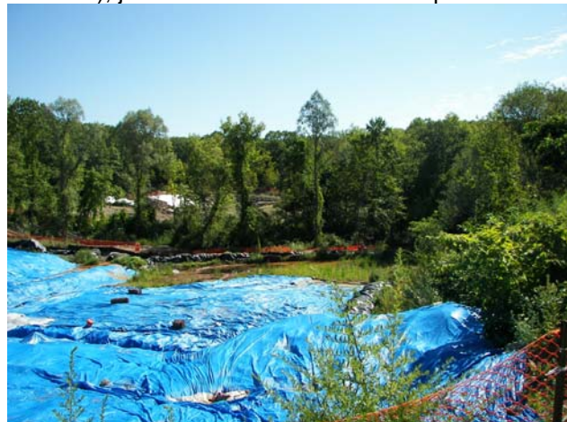
Figure 2. Removal activity at SR-3 (sludge removal area 3), just north of the O'Connor Disposal Area.
