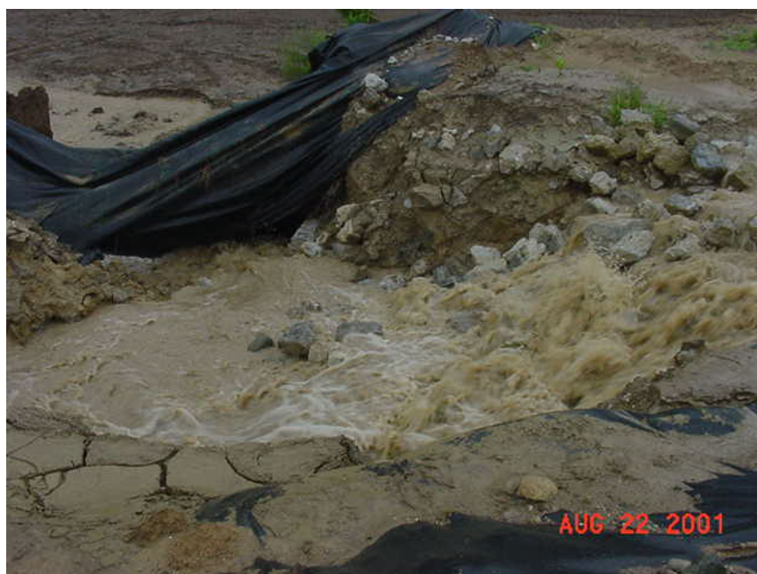
Photo 1: Improperly installed silt fence
