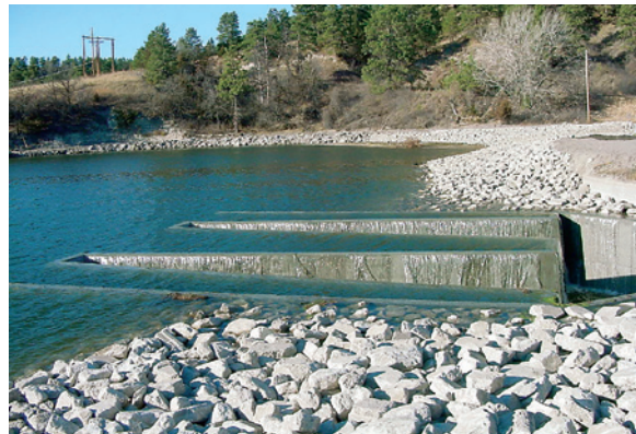
As part of the project, a unique labyrinth spillway was constructed to pass large storm event flows without manual operation. The hydrosuction system passes around the dam shown here.
