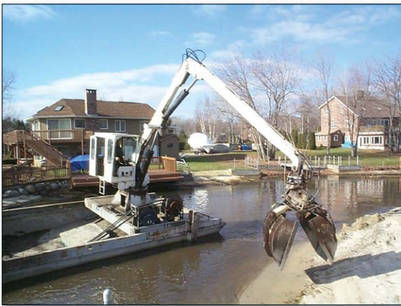
Figure 2: Dredge removing accumulated sediment from the mouth of Middle Brook Canal (Fall 2004).
