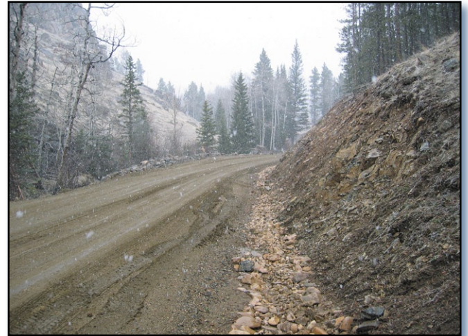
Figure 3. A newly-constructed ditch along the road conveys water away from stream and into a sediment basin.
