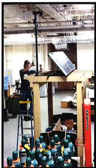
The Village Green station for the Children's Garden location is currently in the fabrication process at EPA.
