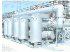
Gas Insulated Substation
