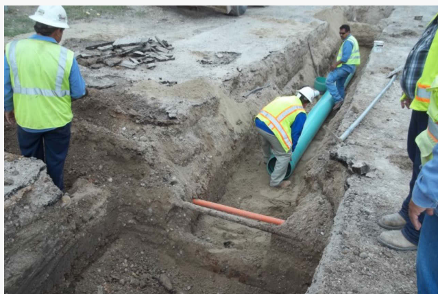
Replacement of wastewater collection line in Rio Grande City, Texas (photo courtesy of NADB)
