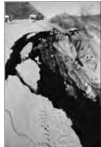
Subsidence, slippage, and other kinds of slope failure can damage structures.
