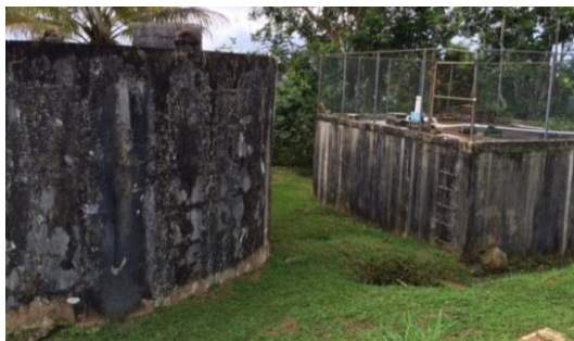
Drinking water storage tanks in a community water system in Puerto Rico that lack functioning chlorination equipment. (EPA OIG photo)
