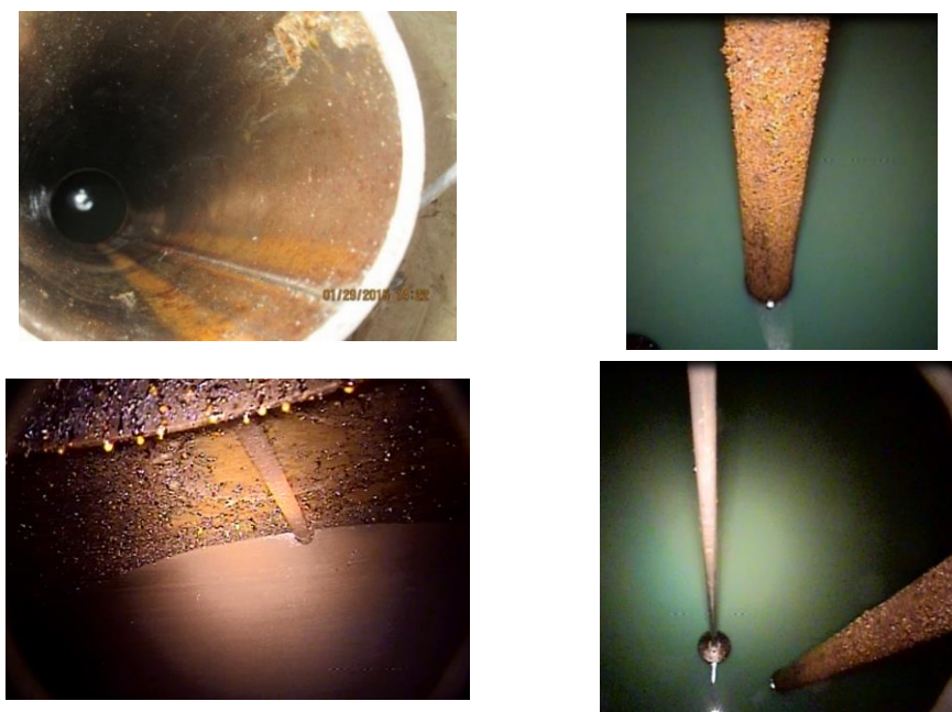
Figure 9. UST System With Steel Tank With Severe Metal Corrosion (43-MD-ST: Installed 1992; Age Of Filter Unknown). Top Left: Fill Pipe Opening; Top Right: STP Shaft; Bottom Left: Tank Top Showing Manway; Bottom Right: ATG Probe And STP Shaft
