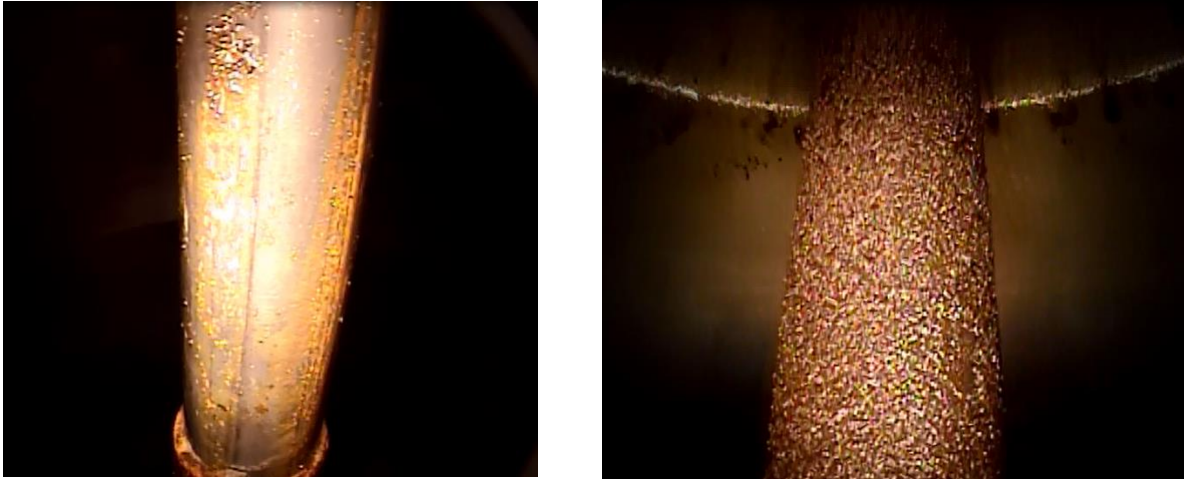
Figure 5. UST System 9-IN-FG STP Shaft Corrosion (Left Photo: Middle Of Shaft [Generally Submersed], Right Photo: Top Of Shaft [Generally Exposed To Air])
