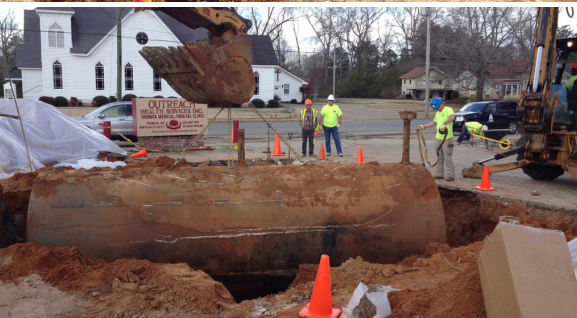
An underground storage tank is excavated from the site of the Shubuta Outreach Family Clinic.
