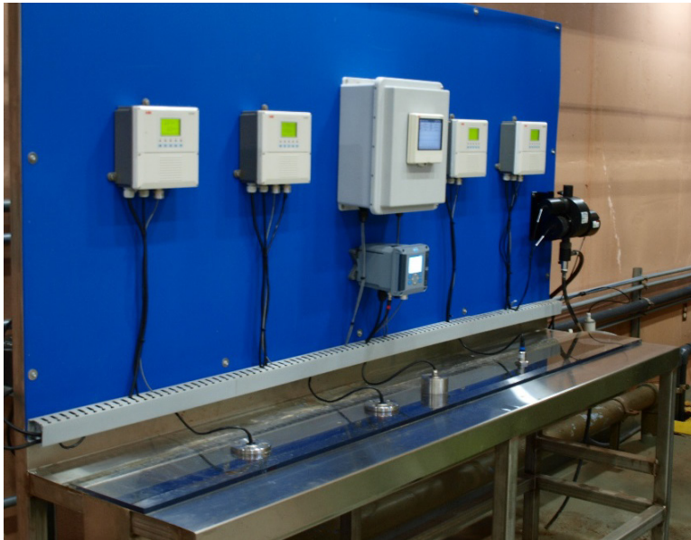
Figure 9-3. West Virginia American Water Monitoring Station
