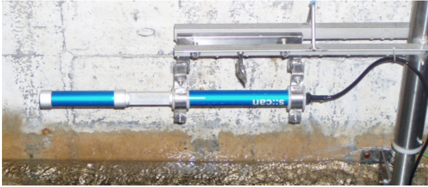
Figure 9-5. Bratislava Water Company Monitoring Station
