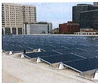
Tulsa's newly renovated downtown library will have a number of public charging stations. The chargers will be partially powered by a solar array on the library's roof.
