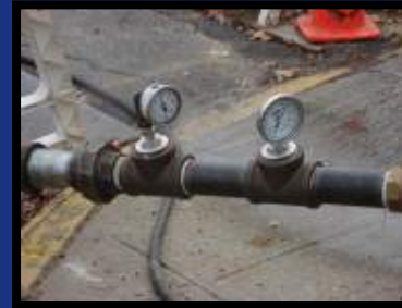
Temperature and Pressure Control
