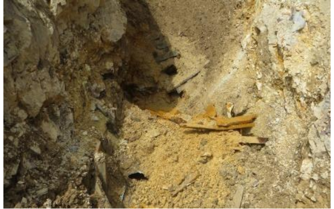
Exposed, collapsed timbers and material filled in and around the timbers at the Gold King Mine portal on the afternoon of August 4, 2015. (EPA photo)
