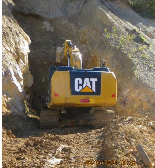
Photo of excavation activities on August 5, 2015. Image was taken about 1.5 hours before the release. (EPA photo)
