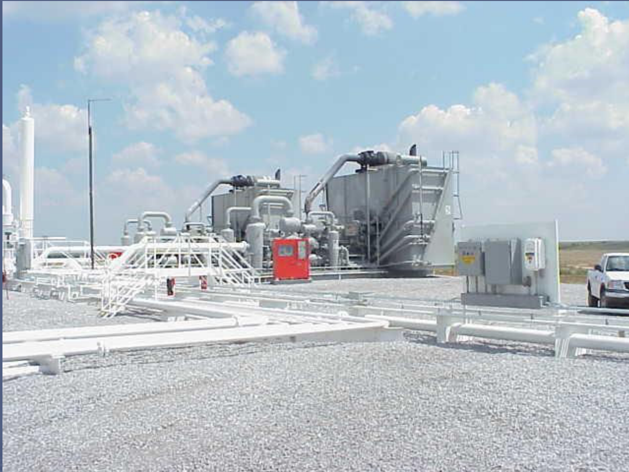
Skid Mounted Compressors
