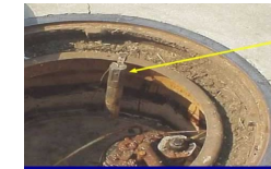
Tank top sump sensor installed too high
