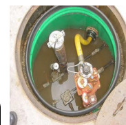
Tank top sump full of liquid
