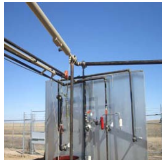
EnCana JATCO Installations in the DJ Basin
