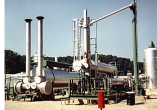
Glycol Dehydrator Unit Source: GasTech
