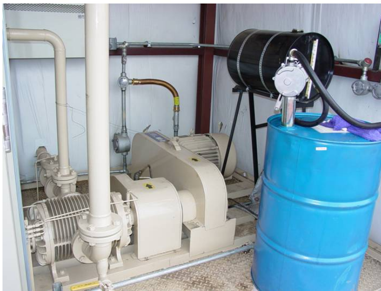
Baker, MT ConocoPhillips VRU installation; Picture Courtesy of Hy-bon Engineering
