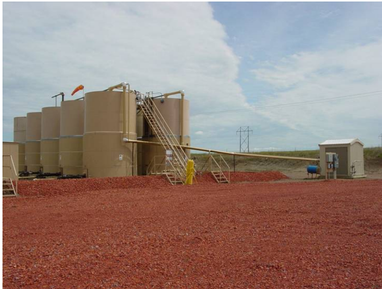
Baker, MT ConocoPhillips VRU installation; Picture Courtesy of Hy-bon Engineering
