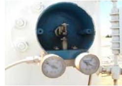
Invalco 415, 215, 402 Retrofit w/ Mizer valve, block & gauges
