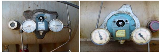
Cemco/WellMark 6900 Retrofit w/ Mizer Valve
