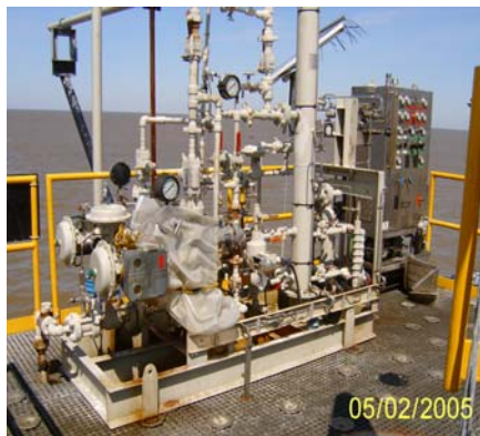
Natural Gas Supply Skid
