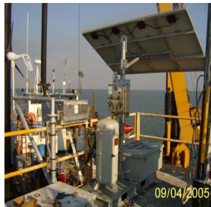
24VDC Compressed Air Supply
