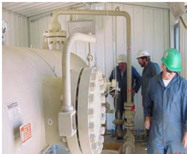
Portable Three Phase Separator, Source: BP
