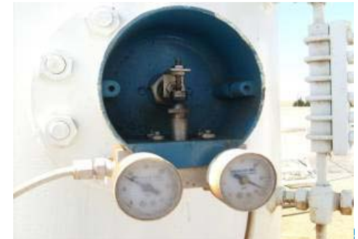
Invalco 415, 215, 402 Retrofit w/ Mizer valve, block & gauges
