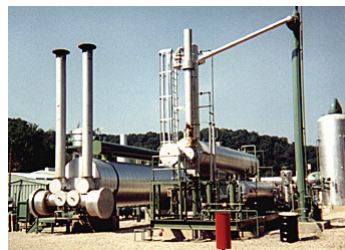
Glycol Dehydrator Unit Source: GasTech
