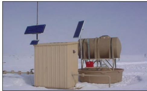
Source: Western Gas Resources
