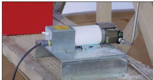
Source: Western Gas Resources
