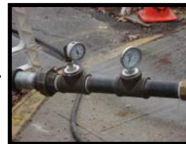
Temperature and Pressure Control
