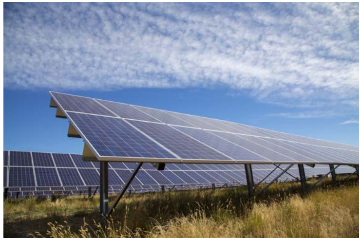
Completed Riverside Community Solar Project at the former defunct Dreher Pickle Plant site. Photo credit City of Fort Collins.
