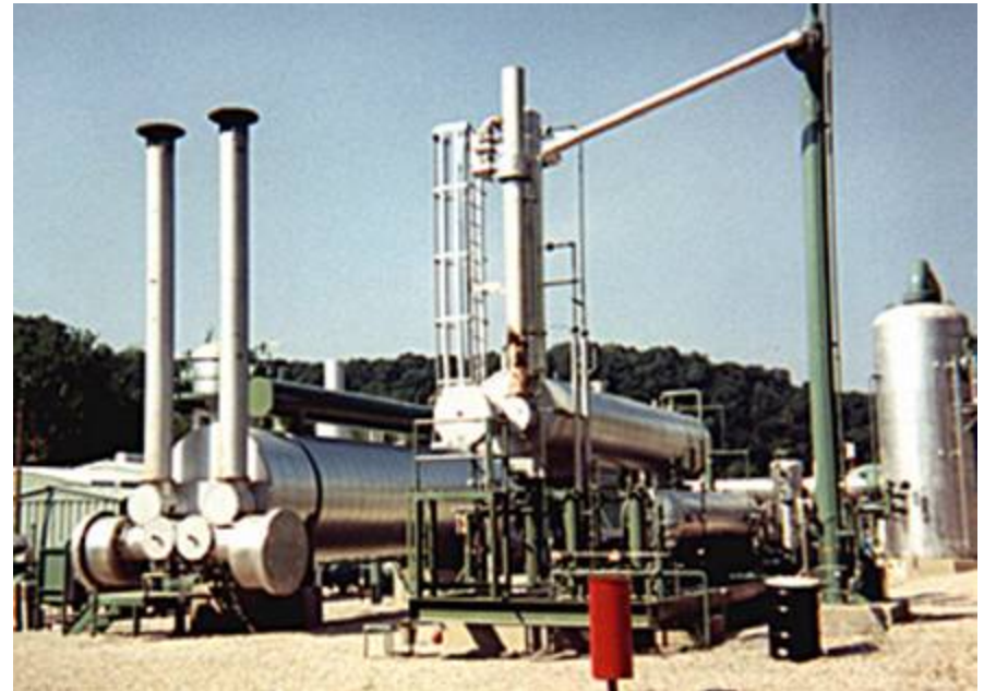
Glycol Dehydrator Unit Source: GasTech
