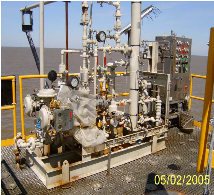
Natural Gas Supply Skid
