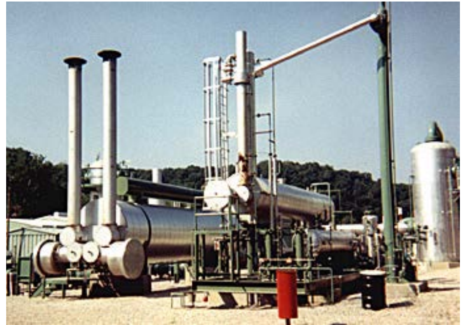
Glycol Dehydrator Unit Source: GasTech
