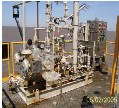
Natural Gas Supply Skid
